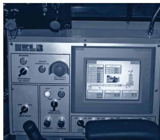
Control panel for deck cranes
